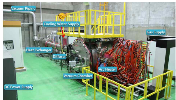
Fig. 1. A Layout of 0.4 MW class supersonic plasma wind tunnel constructed at CBNU (Chonbuk National University)
