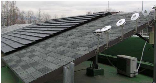
Fig. 2 2kW grid-connected PV system
