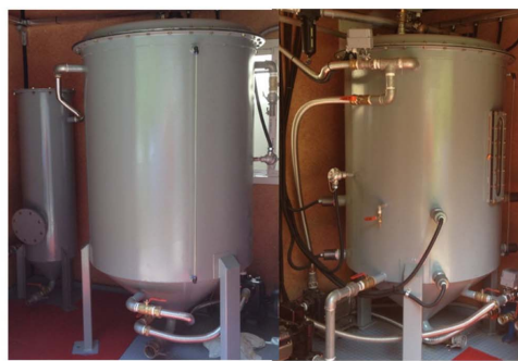
(a) Heating & Water Sparging Remediation System
