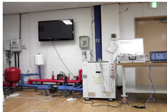
Figure 2. View of a ground source heat pump system
