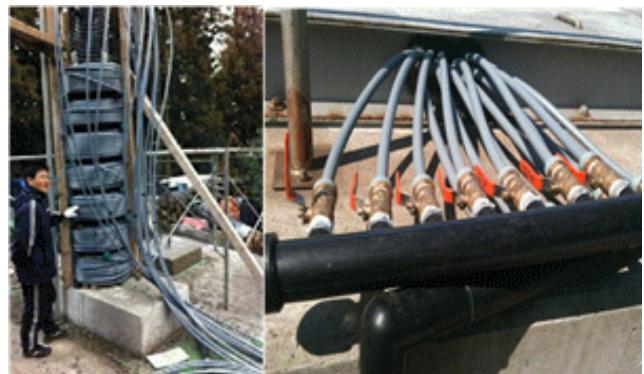
Figure 1. Photo of the PE pipe type heat exchanger.
