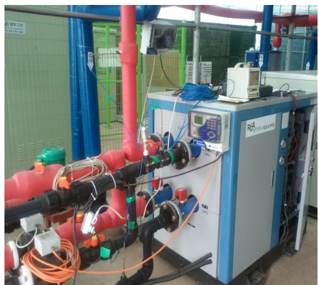
Figure 2. Photo of the water-water heat pump system of 100 kW scale for cooling performance test.
