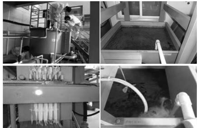
Fig. 1. Treatment equipments of uranium-containing wastewater; A) Neutralizing equipment, B) Separator, C) Filter press, D) Reclaimed water storage tank.
