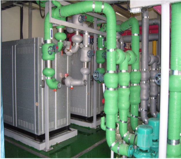
Figure 4. Photo of the system and the pipelines.
