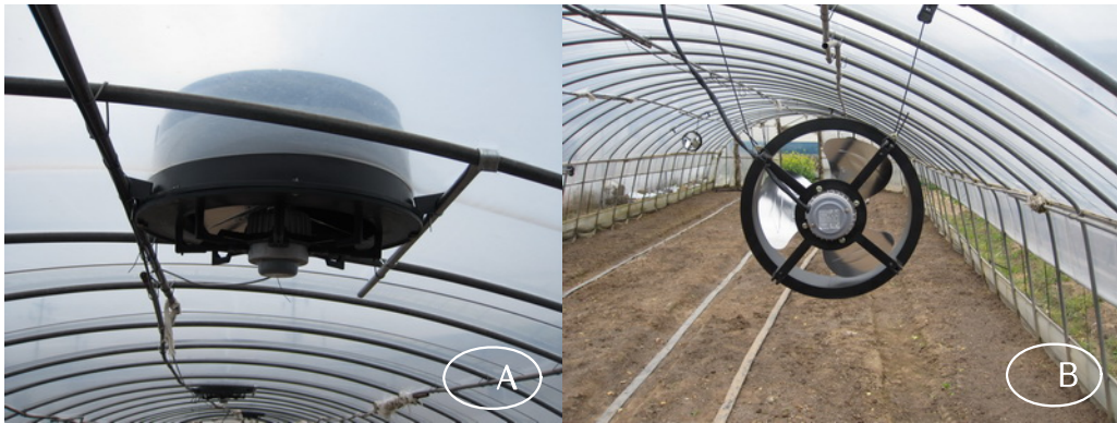
Fig. 1. Installation of vertical forced ventilation fan (A) and horizontal air circulation fan (B) in greenhouse
