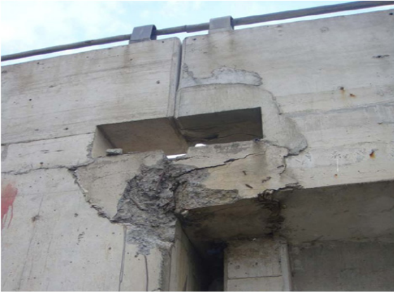
Fig. 1. Pounding between girders of Puente Las Ballenas in 2010 Chile earthquake
