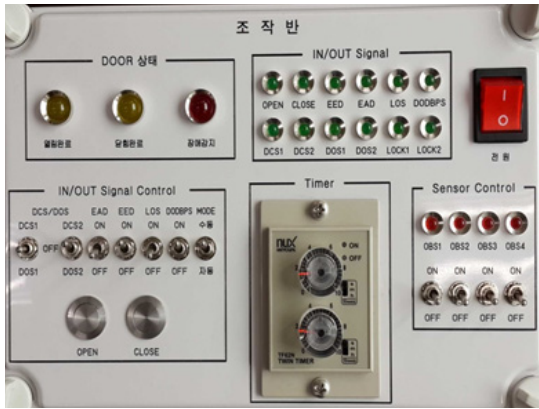
Figure 7. RPSD panel for test operation
