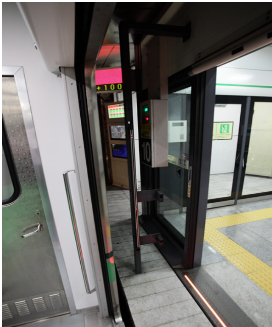
Figure 2. Electrical sensors for detecting obstacles between train door and platform screen door
