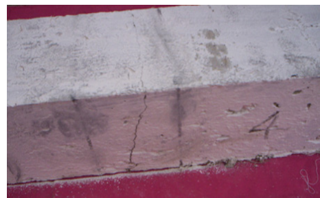
Fig. 15. Crack pattern for coconut fiber added concrete
