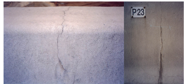
(a) Cracking in horizontal and vertical directions
