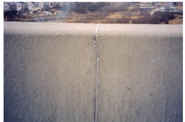
(b) Sealant in crack inducing joint
