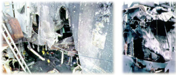
Fig. 1 Internal explosion damage of USS Stark (FFG-31) by Exocet missiles during Iran-Iraq War
