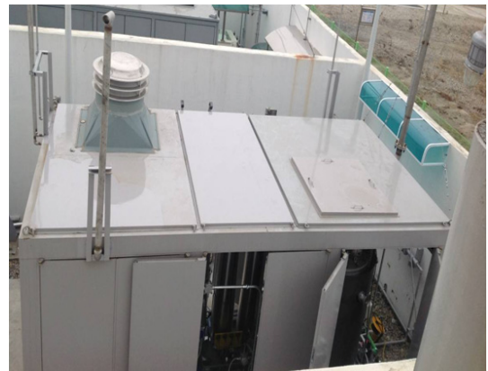
Fig. 1 Appearance of hydrogen generation system for HCNG fueling station
