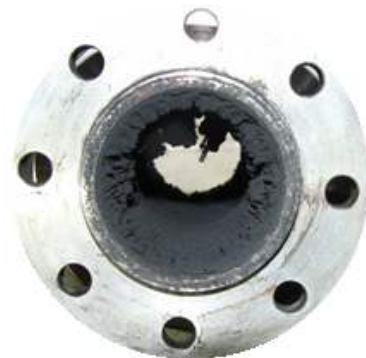
Fig. 8. Soot deposition in the post chamber
