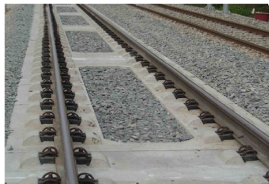
Fig. 1 Photo of continuous welded rail (CWR)
