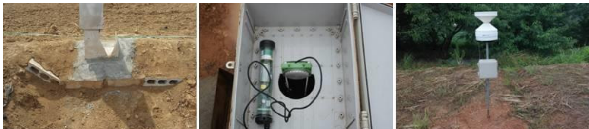
Fig. 3 Installed monitoring equipments (flume, water gage, rain gage)
