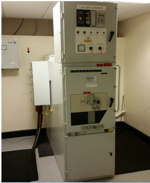
[Fig. 1] VCB panel of High Voltage Generator in Warsash Maritime Academy
