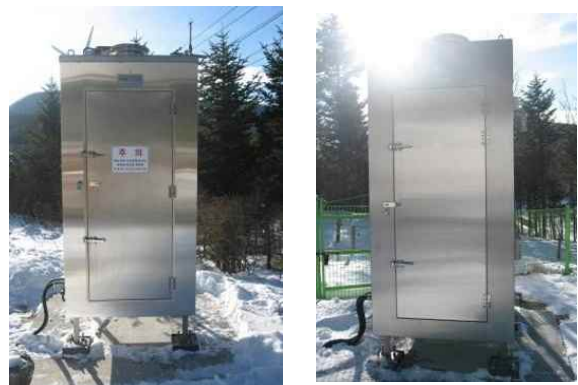
Fig.4. Installed machinery for cloud Observations
