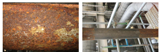
Fig. 1. Corrosion Under Insulation in petrochemical Pipeline.
