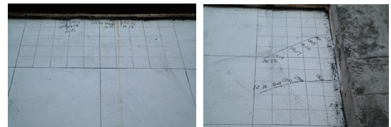
Fig. 15. Cracks on shrinkage restricted concrete wall without w/o using shrinkage reducing agent
