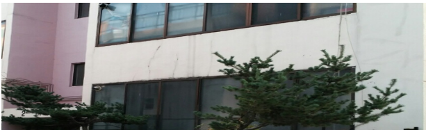
Fig. 3. Poor insulation of old aged apartment
