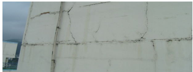
Fig. 4. Crack of old aged apartment
