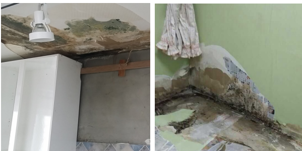
Fig. 2. Water leak and condensation of old aged apartment
