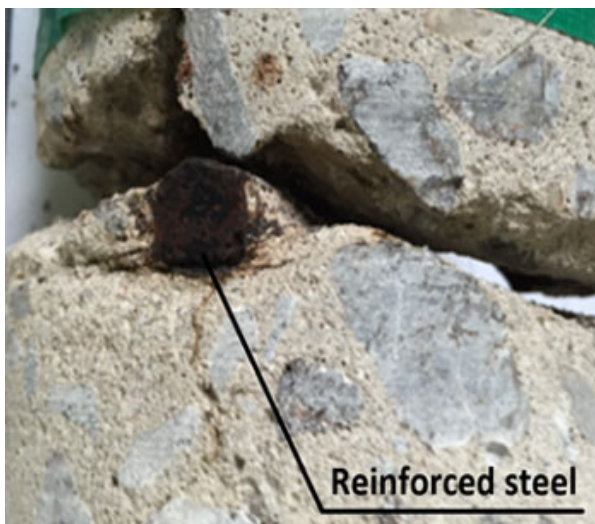
Fig. 13 Crack of Bridge Connection Slab due to Expansion of Reactant around Reinforced Steel
