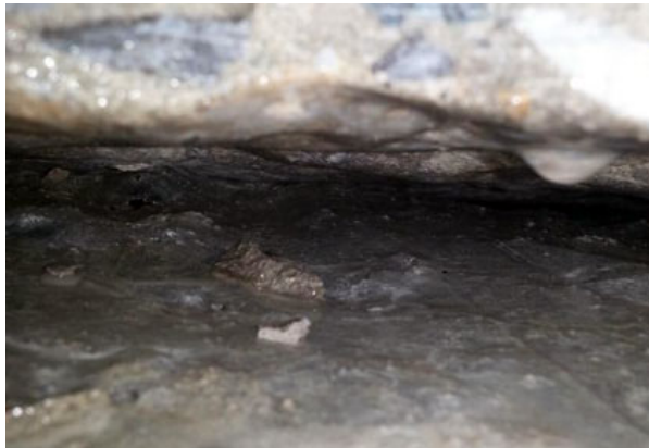
Fig. 8 Cavity between Slab and Subbase in Bridge Connection
