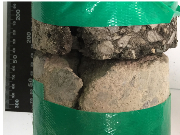
Fig. 9 Through Crack in Asphalt Overlay Pavement
