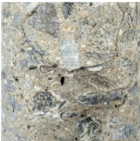
Fig. 5 White Gel and Crack Caused by ASR
