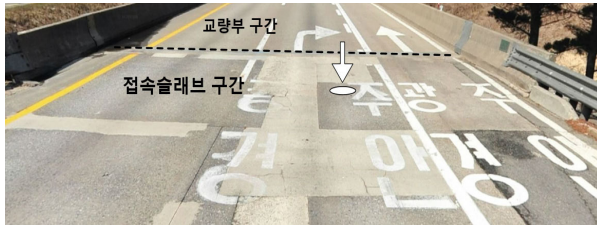
Fig. 7 Distress of Bridge Connection Pavement
