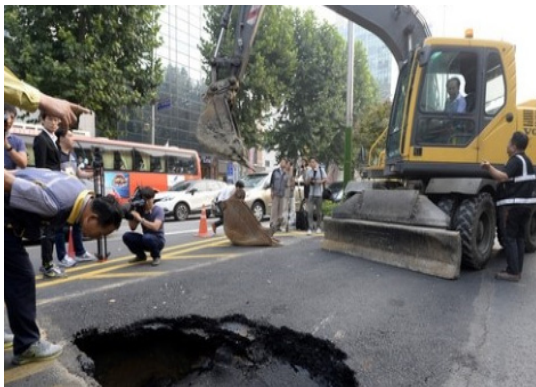
Fig. 2. Road subsidence caused by pipe damages
