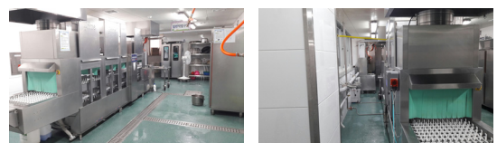
Fig. 9. Dish washing area
