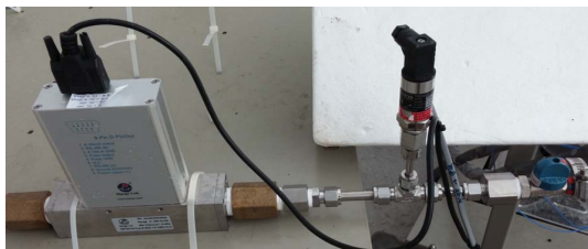
Fig. 3. Installation of flowmeter and pressure gauge.
