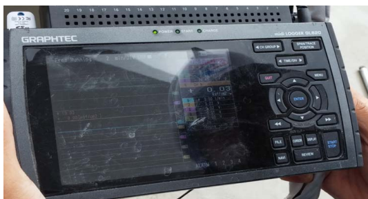
Fig. 4. Data logger for flow, pressure, wind direction and wind speed.
