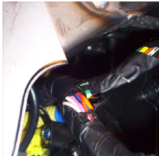
Fig. 8. Damaged wiring example of crash pad lower side.
