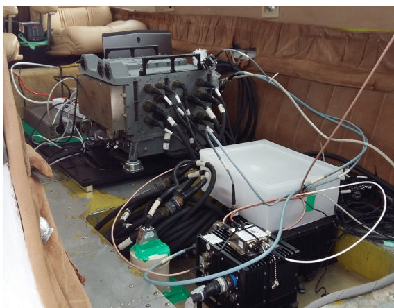
Fig. 5. Equipment installed in the cabin
