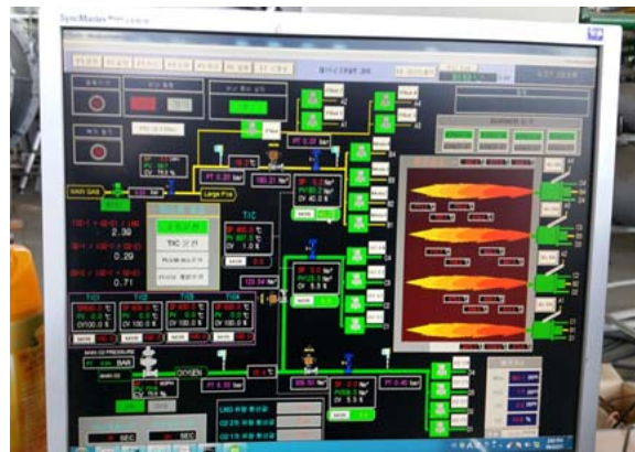
(B) HMI Screen for Control of Ambient Temperature
