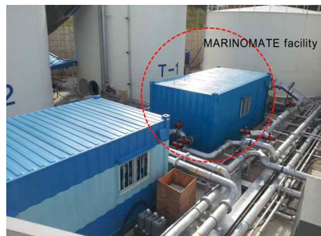
Fig. 7 Electrolysis ballast water treatment system
