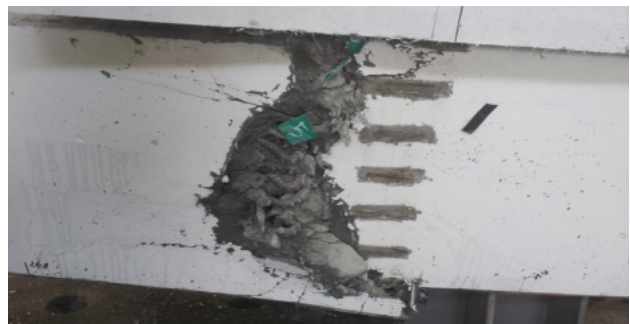
Fig. 17. Failure pattern of UFS1.0
