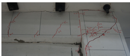
Fig. 8 Crack between beam and slab
