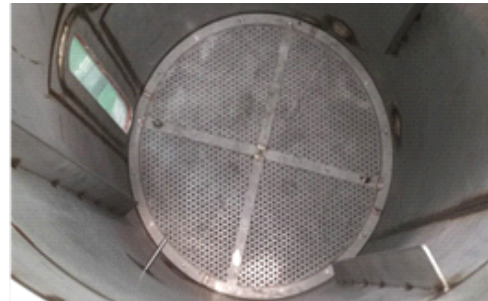
Fig. 4. Screen mesh installed in biodiesel reactor.
