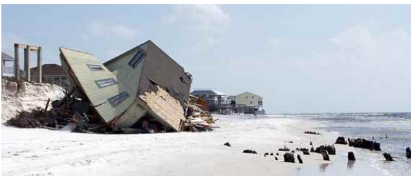
Fig. 3 Lee county damage case1
