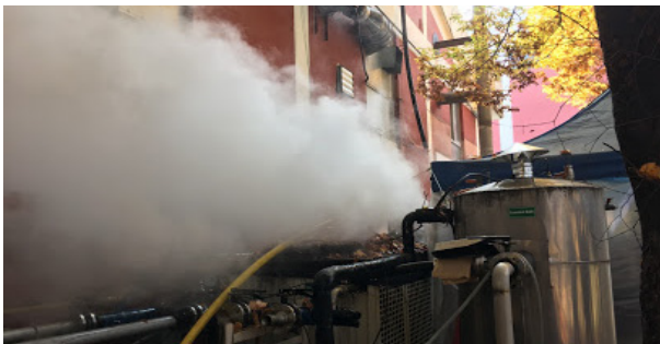
Fig. 5 State of steam generation.
