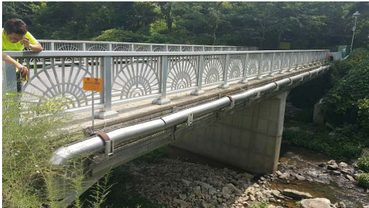
Fig. 1. A typical example of city gas pipe install- ed on the bridge.
