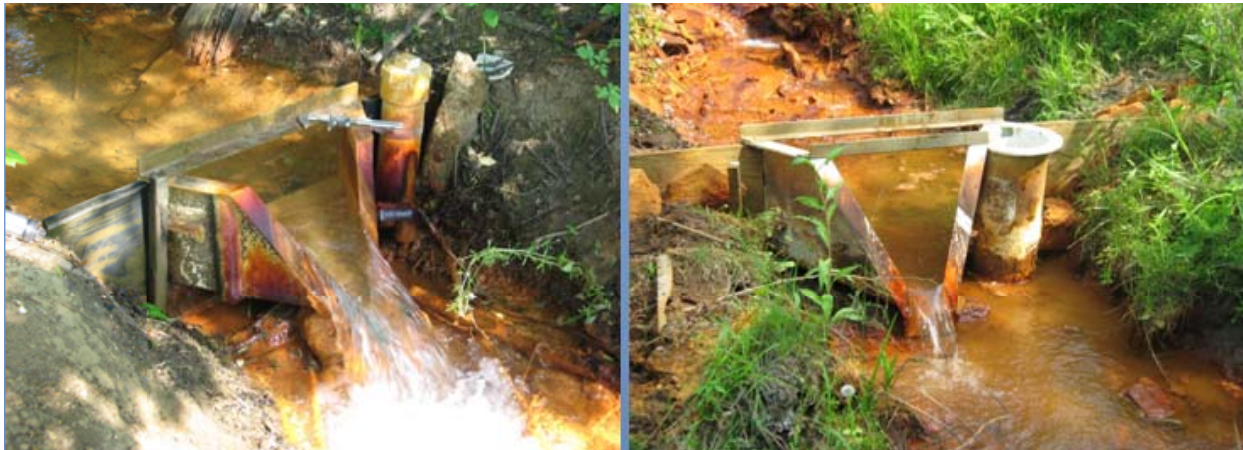
Figure 7. (a) H-Flume at the Primrose discharge, (b) H-Flume at the Hopper discharge
