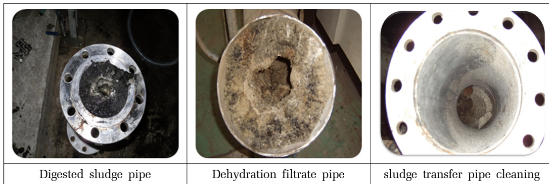
Fig. 3. Field struvite generation piping appearance.
