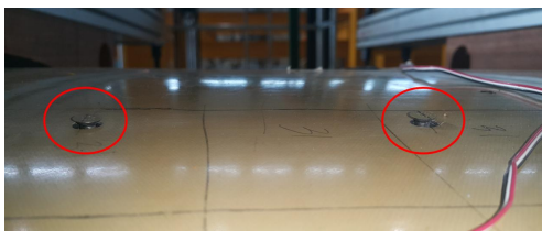
Fig. 14. Fastener pull-through due to buckling
