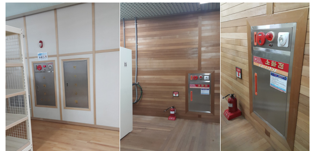
Figure 9. Cases of indoor hydrant installed at museum storage.
