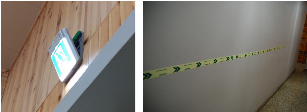
Figure 14. Cases of exit signs (left) and evacuation line installation (right) inside museum storage.
