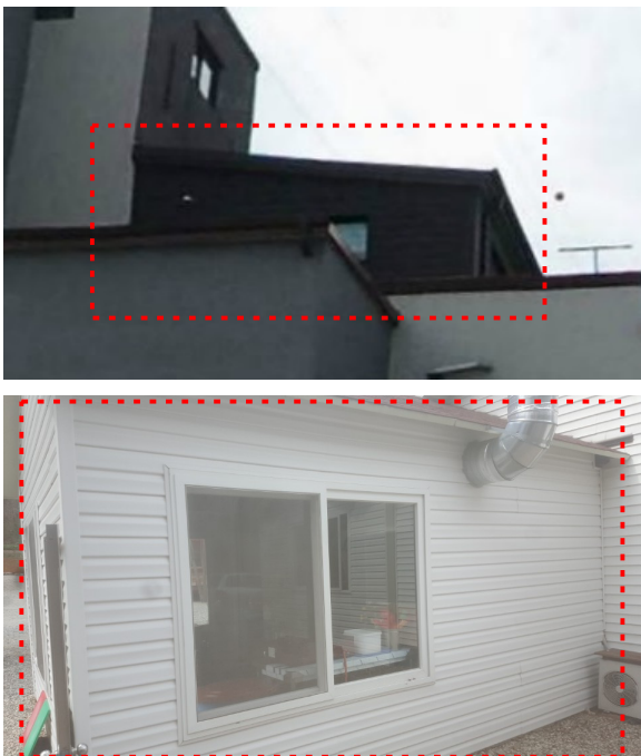
Figure 4. Example of illegal extension.
