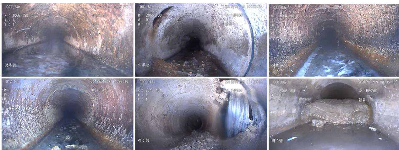
Fig. 2. Condition of sanitary sewer in a part of Seoul in January 2018.
