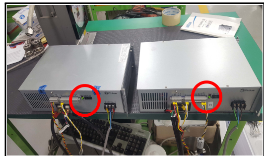
Fig. 9. The power conditioning system connected grid(before anti-islanding).
