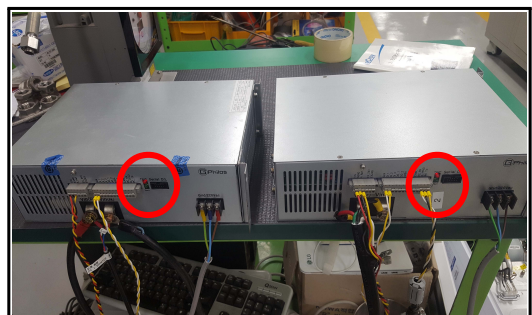
Fig. 10. The power conditioning system connected grid(after anti-islanding).
