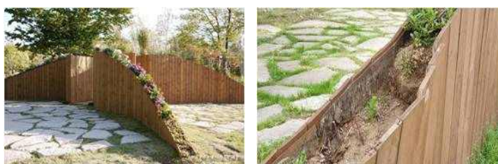
Picture 6. Destroyed Planting Media
