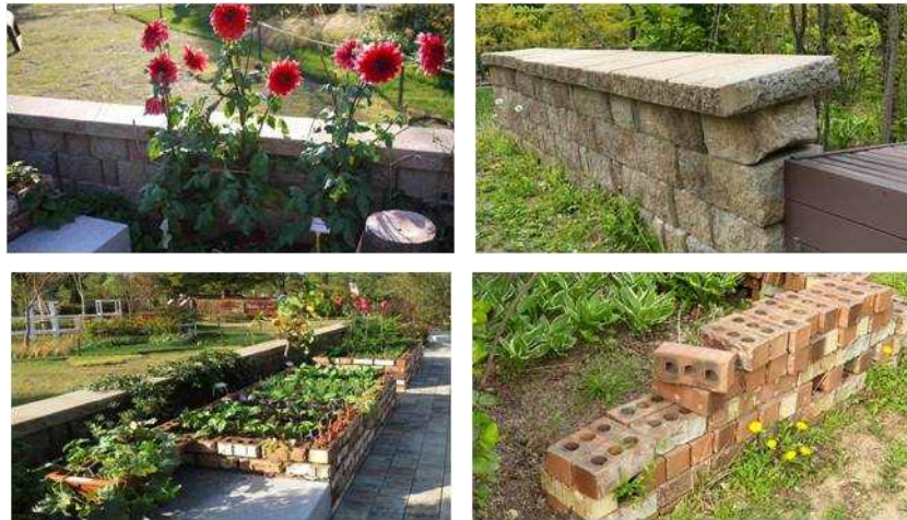
Picture 5. Damaged landscape structure
