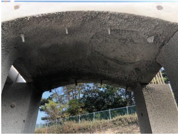
Fig. 7. Dropouts of secondary shotcrete in section 3
