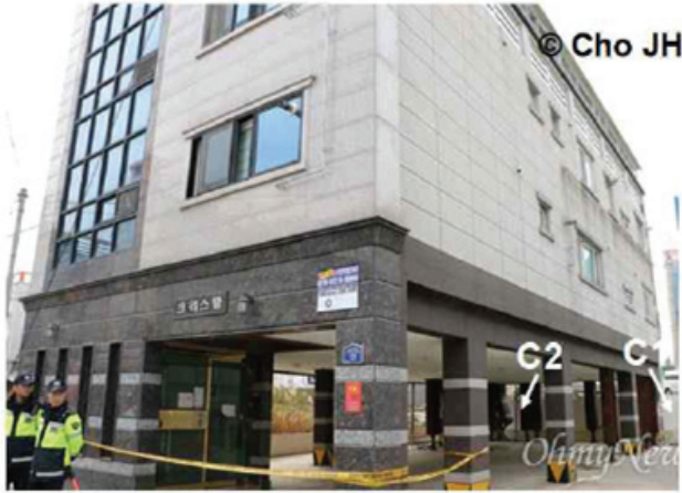
Photo 1 Seismic Damage of Irregular Pilotis Building (Lee, 2018)
