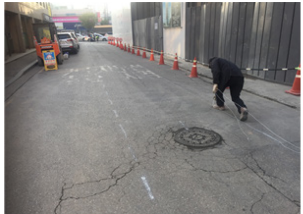
Fig. 5. Marking about Cutting Road
