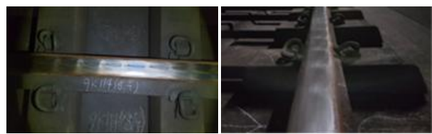
(a) Rail corrugation
