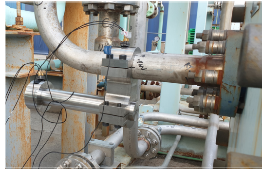
Fig. 13. (Color available online) TMD installed on pipe system.
