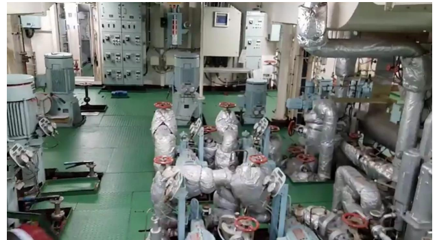
Fig. 5. Target monitoring site in vessel engine room.
